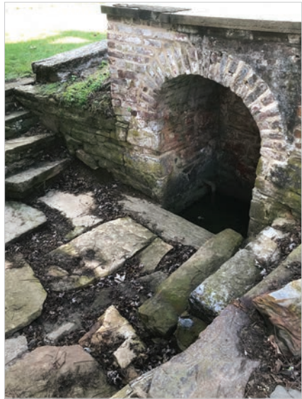
Figure 2.22 Still-Flowing Spring. The steps shown here lead to a spring that flowed during the Battle of Antietam—and it is still flowing. Natural springs were vital to farms and homesteads, and they were lifesaving necessities when tending to the wounded. Courtesy of Scott C. Woodard, US Army Medical Department Center of History and Heritage; November 2017.
