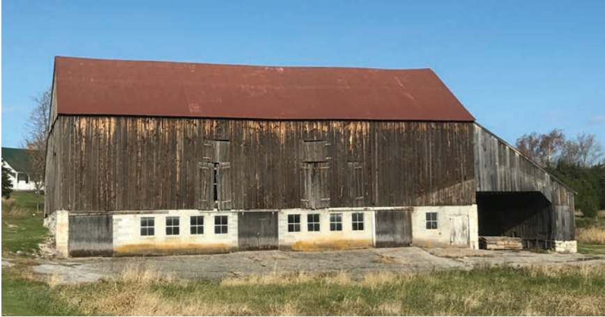
Figure 2.18 Roulette Barn Exterior. The exterior of the Roulette Barn seen from the east coming from Bloody Lane at the Antietam National Battlefield. This was the first structure built that offered some protection for the wounded fleeing death at the Sunken Road. Courtesy of Scott C. Woodard, US Army Medical Department Center of History and Heritage; November 2017.
