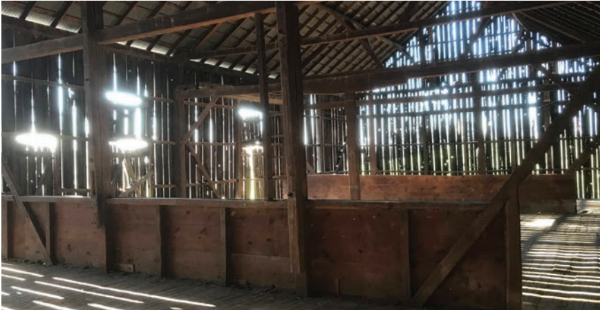
Figure 2.19 Roulette Barn Interior. The interior of the Roulette Barn at the Antietam National Battlefield. Notice how the original frame displays signs of shaping with hand tools. Courtesy of Scott C. Woodard, US Army Medical Department Center of History and Heritage; November 2017.
